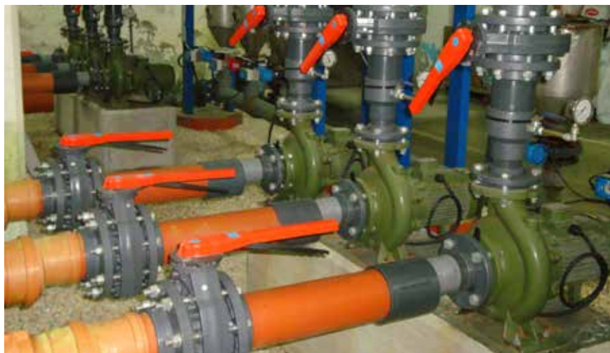
NR. 25 IR4P 65-250NB SPAIN PVC PRODUCTION PLANT
