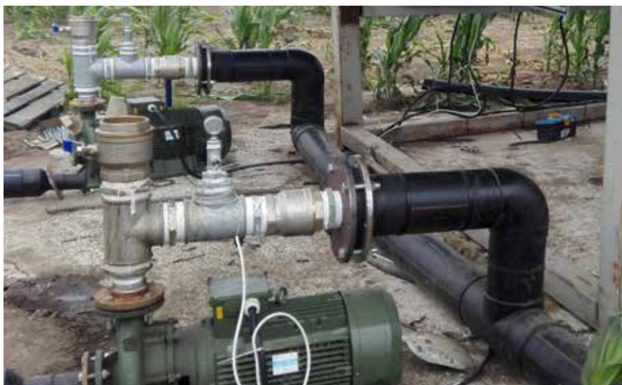
NR. 2 IR 50-250ND with control panel with inverter BULGARIA IRRIGATION IN A CORN FIELD
